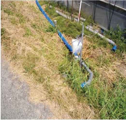
Fig 2.6-f Flow meter (Water tap)
