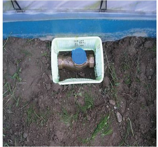
Fig 2.6-g Water meter (Well)
