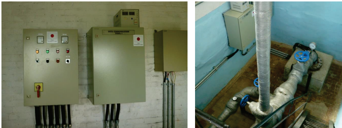
Figure 3.5 Photo of deep-well's inside
